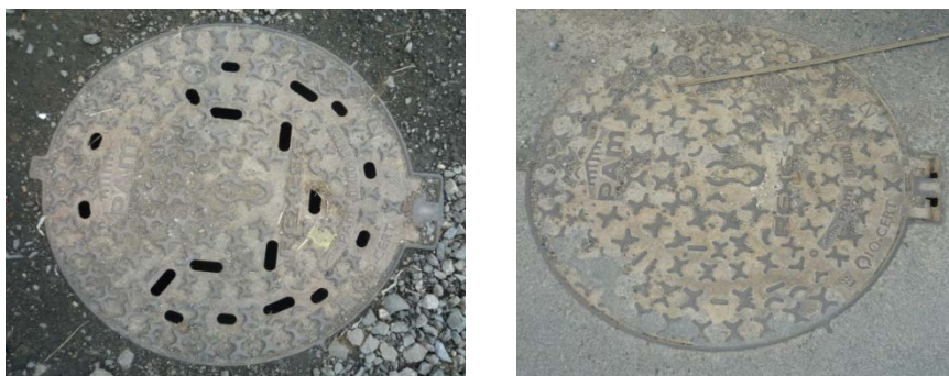
Picture 2 - Covers used in Všeřtary - with venting holes and full covers
